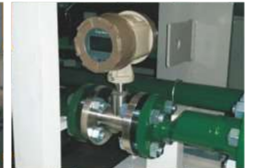
Liquid turbine flowmeter in water supply plant
