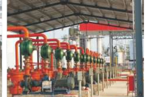
Oval gear flowmeter in petrochemical industry
