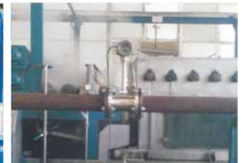
Vortex flowmeter in boiler system for steam measurement
