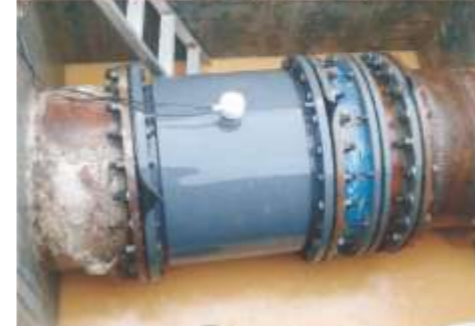
Magnetic flowmeter in under well field
