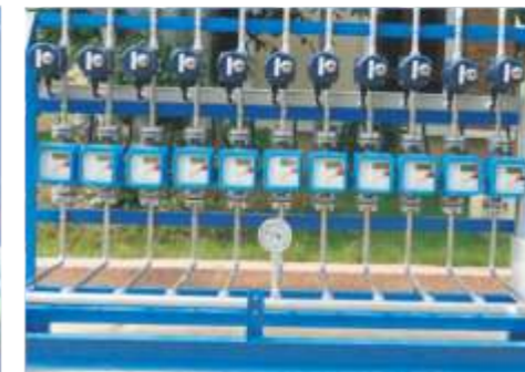
Rotameter system for mixed gas measurement
