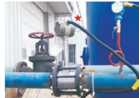
Vortex flowmeter in oxygen measurement
