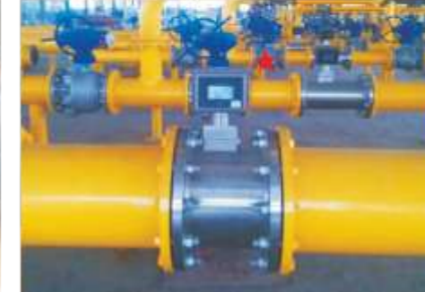
Gas turbine flow meter in nature gas filling field
