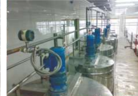
Liquid turbine flowmeter in food and beverage industry
